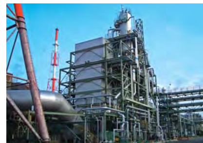
Newly installed exhaust air reheat boiler at the Mizushima plant
